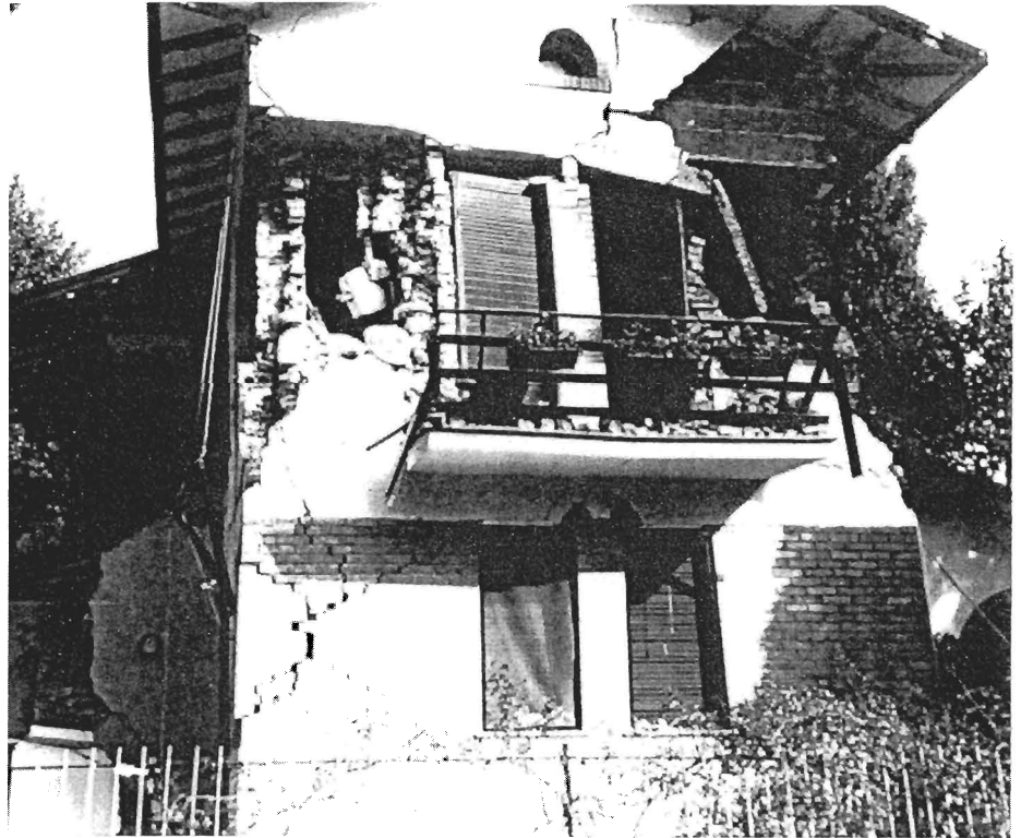
Figure 4 Severe damage to modern house in higher area of Cesi
